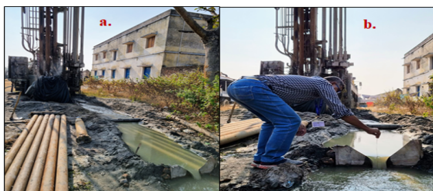
Figure 4: a) Discharge of the bore well during the preliminary yield test at Narrah 4, b) Measurement of discharge using 90° V-notch weir plate.
